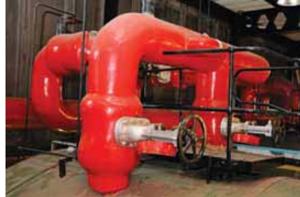
Figure 48 Asbestos-insulated supply pipes
