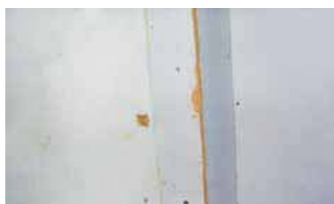
Figure 24 Chrysotile paper on fibreboard boxing
