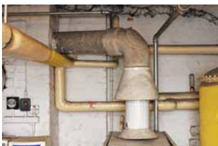
Figure 34 Asbestos cement boiler flue
