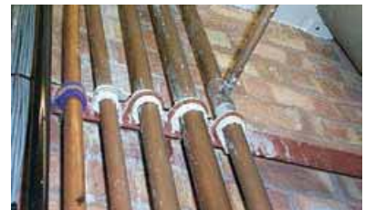
Figure 29 Chrysotile cloth on pipes
