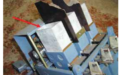
Figure 49 Electrical switchgear with asbestos flash protection
