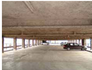
Figure 7 Sprayed limpet on car park roof
