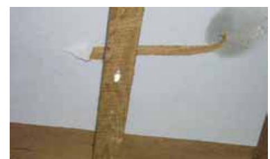
Figure 25 Chrysotile paper on strawboard ceiling panels
