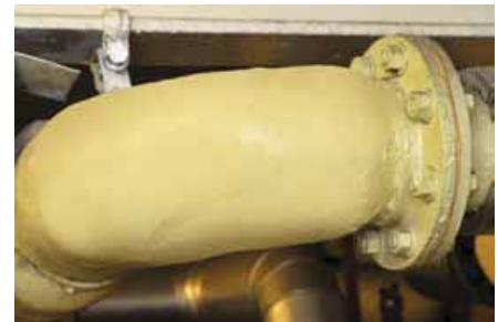
Figure 10 Pipe insulation with coating
